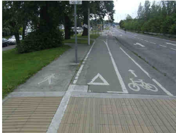
Existing arrangement means pedestrians have to walk on cycle tracks to get to bus stop
